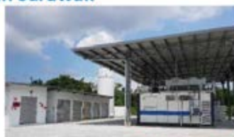
Hydrogen Production Plant
