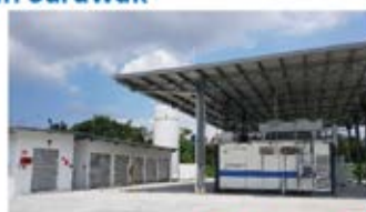
Hydrogen Production Plant
